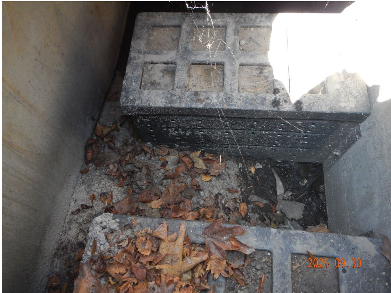
The BioClean Modular Wetlands Linear System chamber is dry, contains pre-filter cartridges and has a moderate buildup of fine sediment and organic litter.
