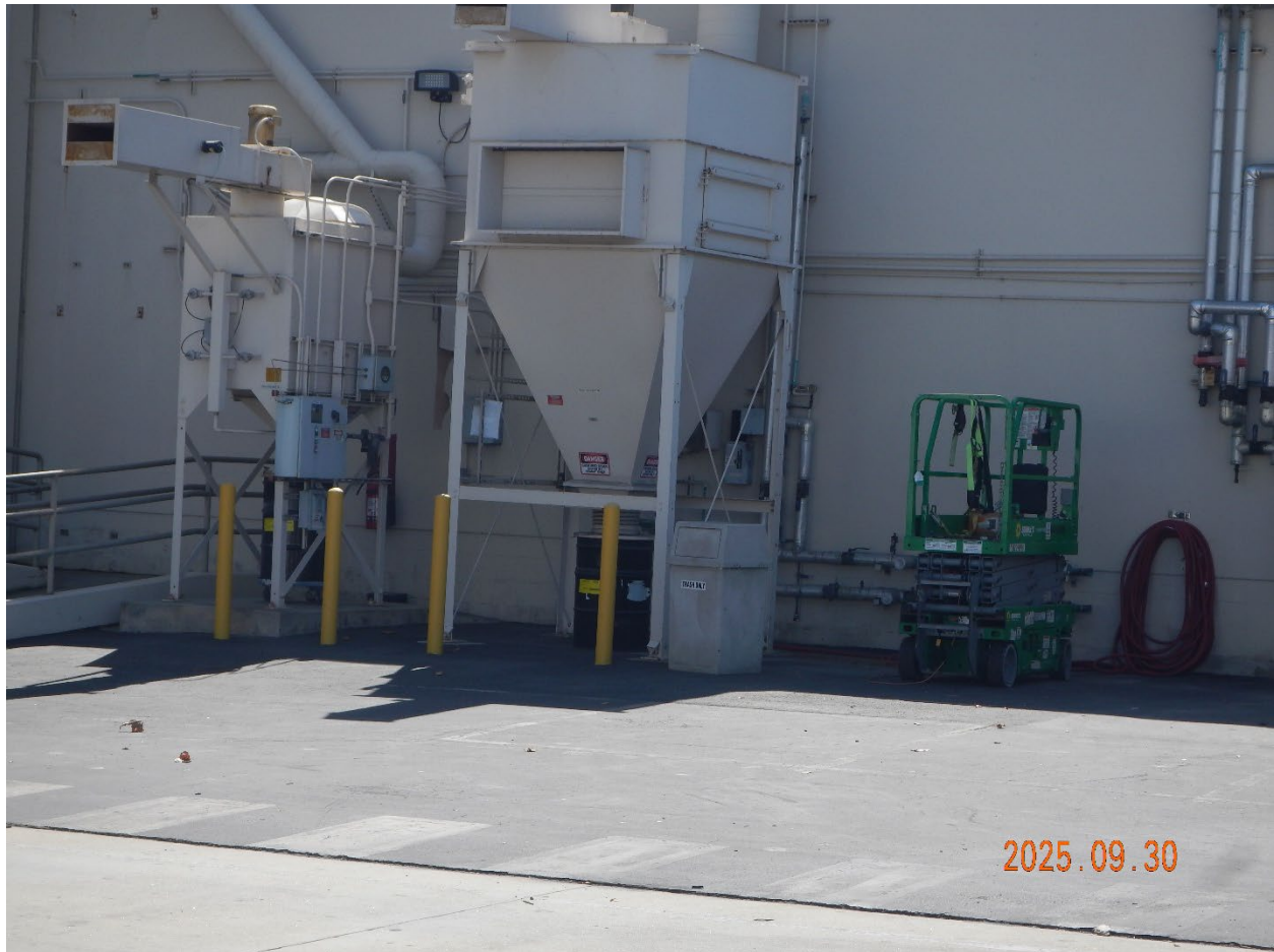
Closer view of the previous photo for the particulate collection system. The red hose on the right of the photo is an air hose.
