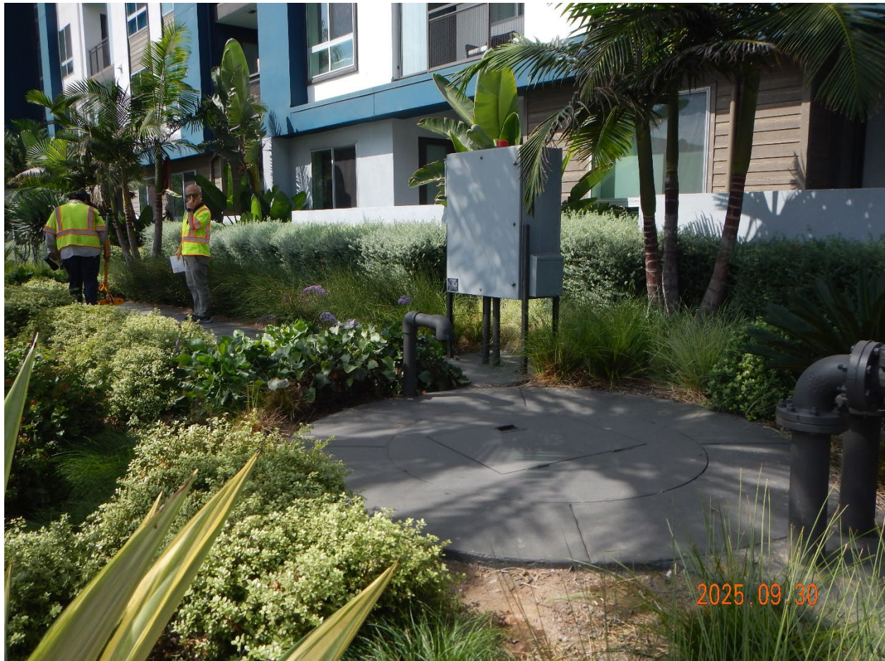
The sump pump control panel for the Contech BioClean Modular Wetland System. Both the pump and the control float valve lights were observed on, indicating that the system was operating.
