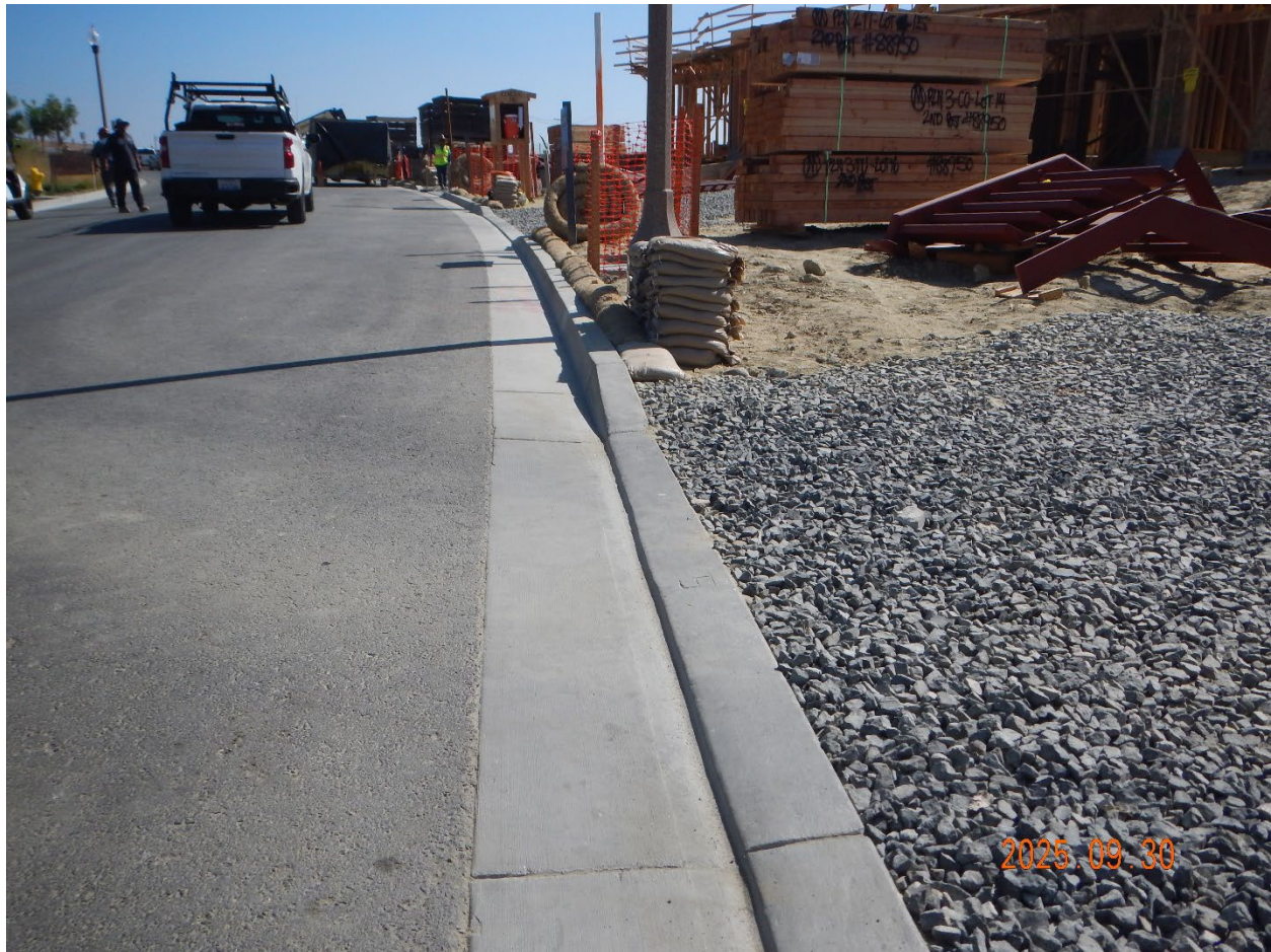
A view of the gravel bed on a residential lot under vertical development, with extra gravel bags added to prevent sediment from leaving, as noted by the superintendent.
