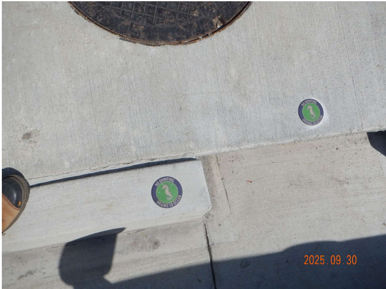
Closer view of the BioClean Modular Wetlands Linear System inlet with medallions.
