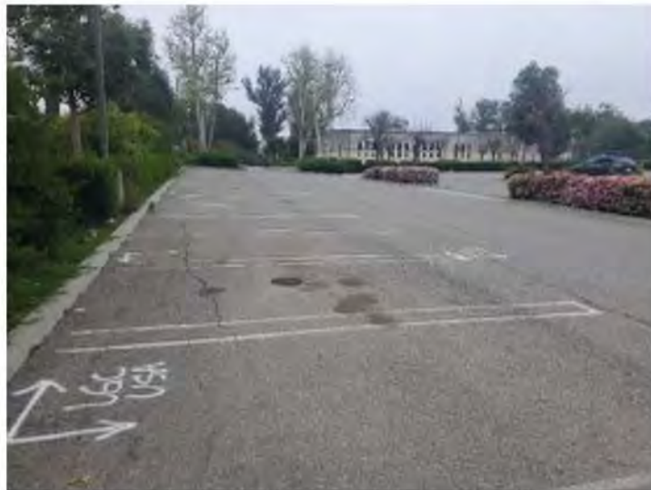
Photograph 10: View of an apparent previous boring performed on the subject property.
