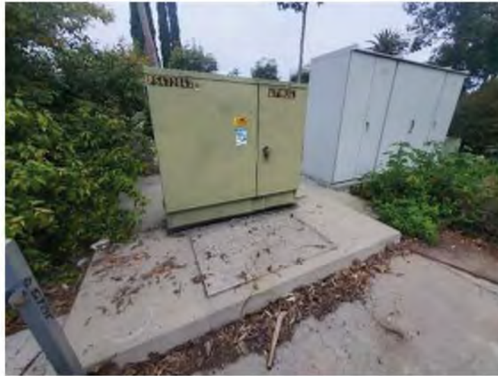
Photograph 11: View of pad mounted transformer on subject property.
