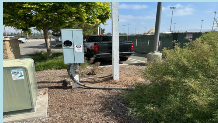
Temporary power poles installed and ready for Edison to inspect and energize for site power
