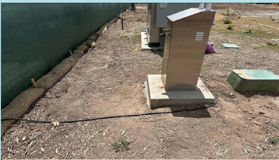
C-8 irrigation control power rerouted to make way for construction
